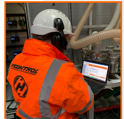
A Hycontrol engineer configures a HMI display via a connected laptop
